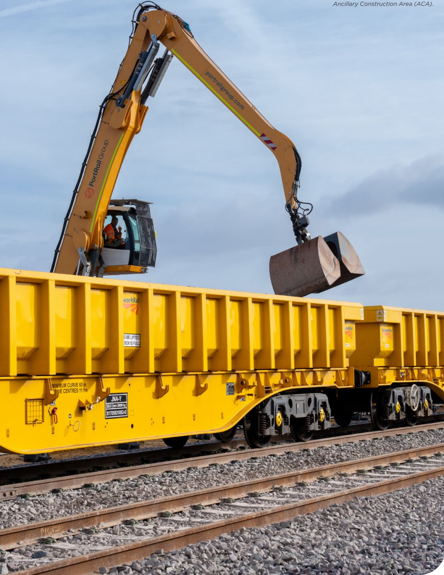
The first engineering trains arrive on site at our Ancillary Construction Area (ACA).
