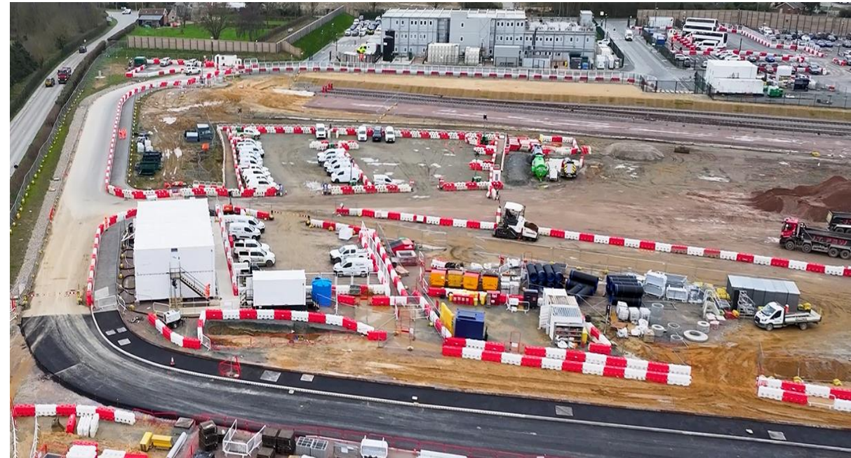
ACA Train line end and storage with rear view of project offices
